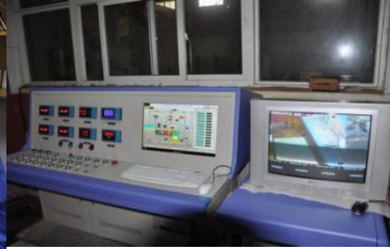
160KW examining and test system
