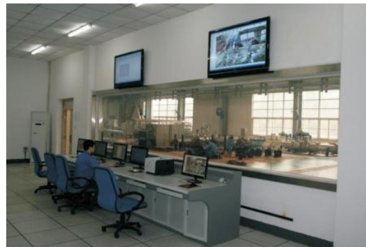
Control room of pump test-bed
