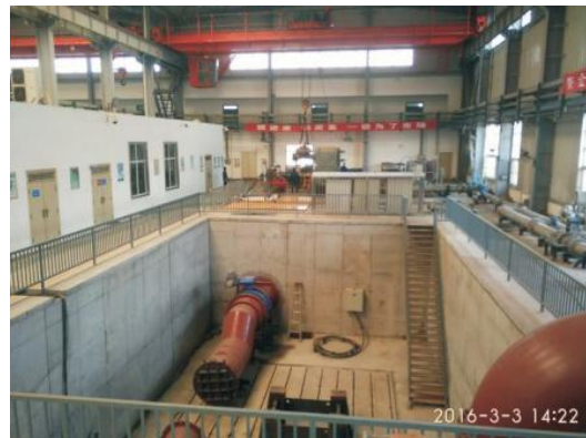
Pump water supply system
